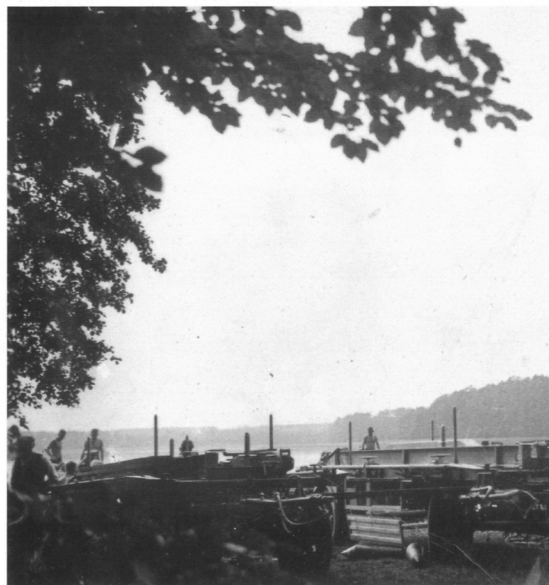
SS engineers erecting a pontoon bridge across the Dnieper River in southern Russia in the late stages of the summer campaign with Heeresgruppe Süd . During September 1943 some 68 German divisions – 1,250,000 men and over 2000 tanks - were withdrawn across the Dnieper river and were tasked with holding the river line at all costs.
