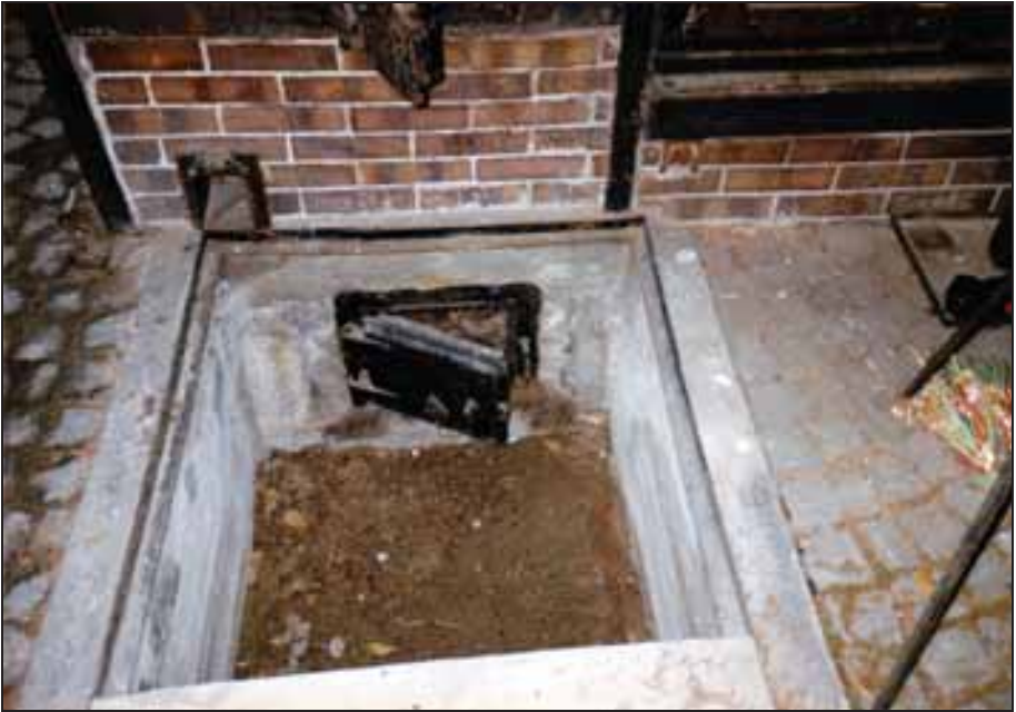
Photograph 7: Left-hand gasifier: slag/ash-removal door and service pit.
