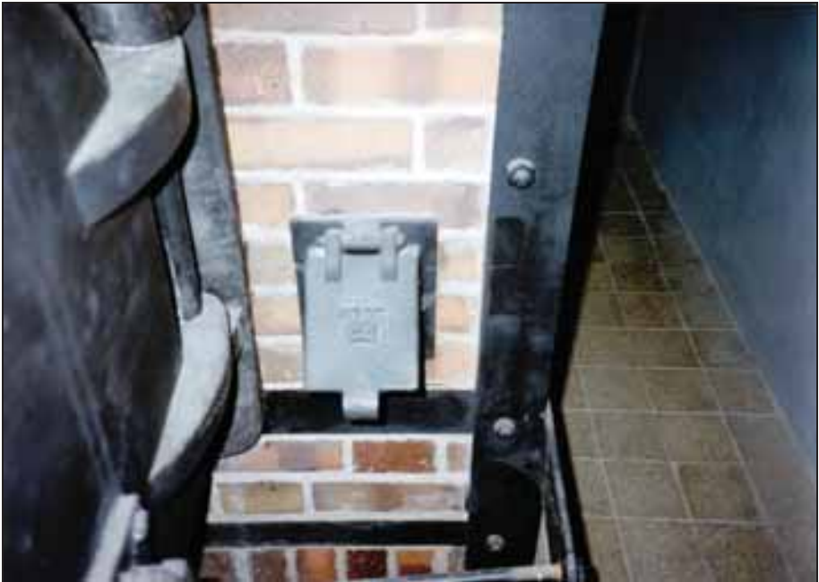
Photograph 59: Door for the combustion-air channel of the right-hand muffle.
