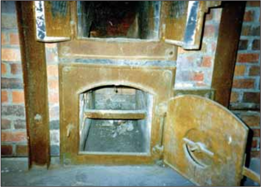
Photograph 262: Ash-chamber door of the main gasifier.
