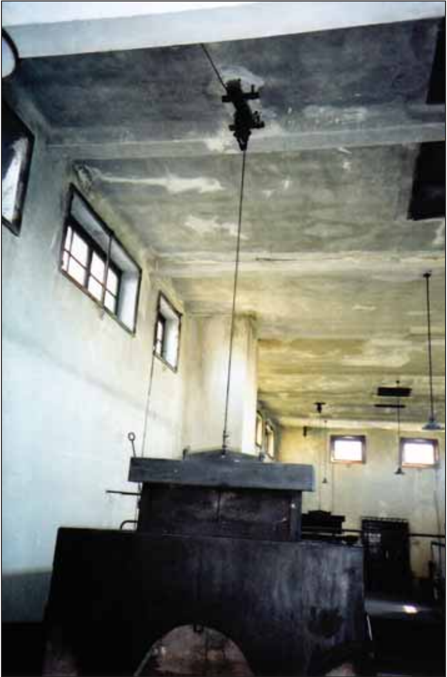
Photograph 360: left-hand furnace of front pair, front view; the damper's steel cable and pulley attached to the ceiling.
