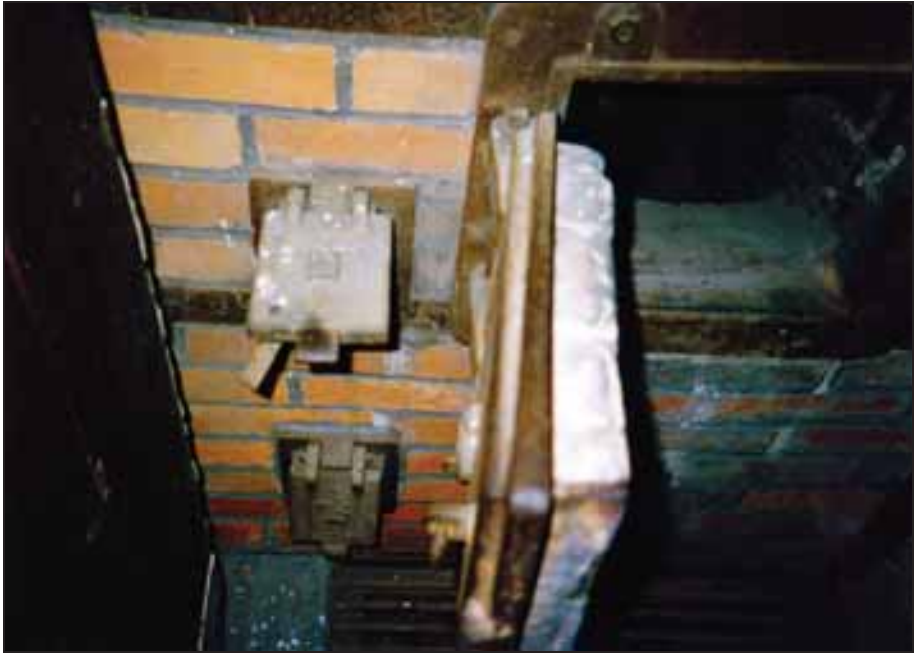
Photograph 39: Left-hand gasifer: large coke-loading door (right), small doors for the primary air to the hearth (bottom) and the primary air to the gasifer (top).
