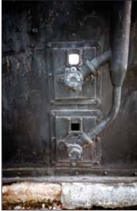
Photograph 333c: rear view, main (top) and auxiliary burner (bottom)
