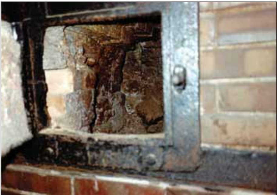
Photograph 9: Right-hand gasifier: coke-loading door.
