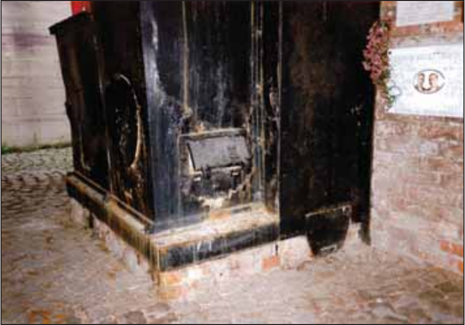
Photograph 34: The rear of the furnace with chimney (left-hand side) with an access door to a pilot flame at the chimney's base. The circular sheet metal welded to the chimney's base closes the original opening for a forced-draft blower.
