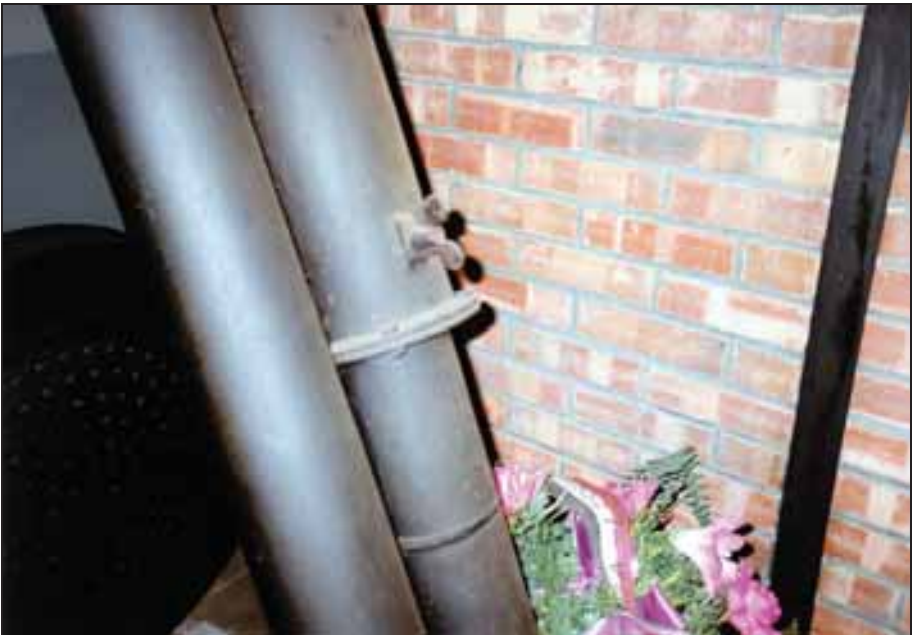
Photograph 194: Tube from the combustion-air blowers to the furnaces; butterfly valve in the right-hand tube for regulating the air flow.
