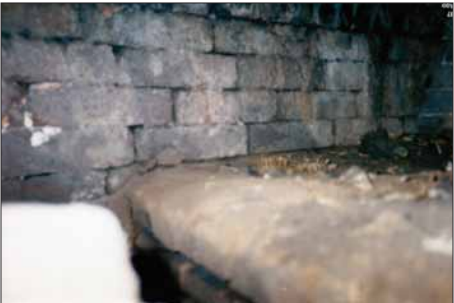
Photograph 282: as above. The muffle's ash chamber seen through the auxiliary gasifier's ash-chamber door.
