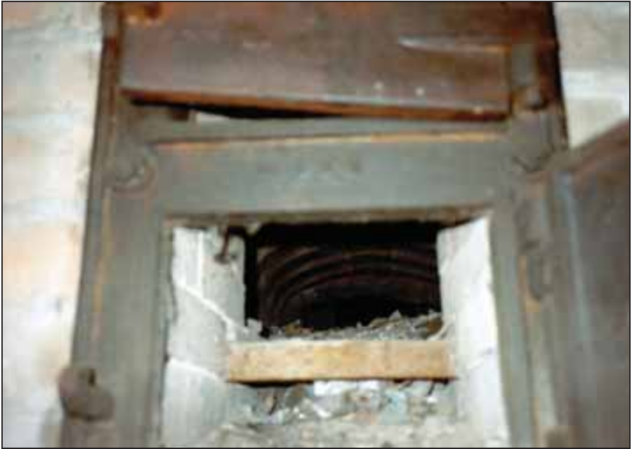
Photograph 304: Ash-extraction door with the first bar of the post-combustion grate visible.
