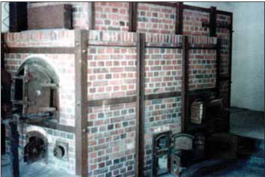
Photograph 257: First furnace, right-hand side: two doors of the auxiliary hearth (center bottom): coke-loading door (rear center), and main-ash-chamber door of the main gasifier (rear bottom).
