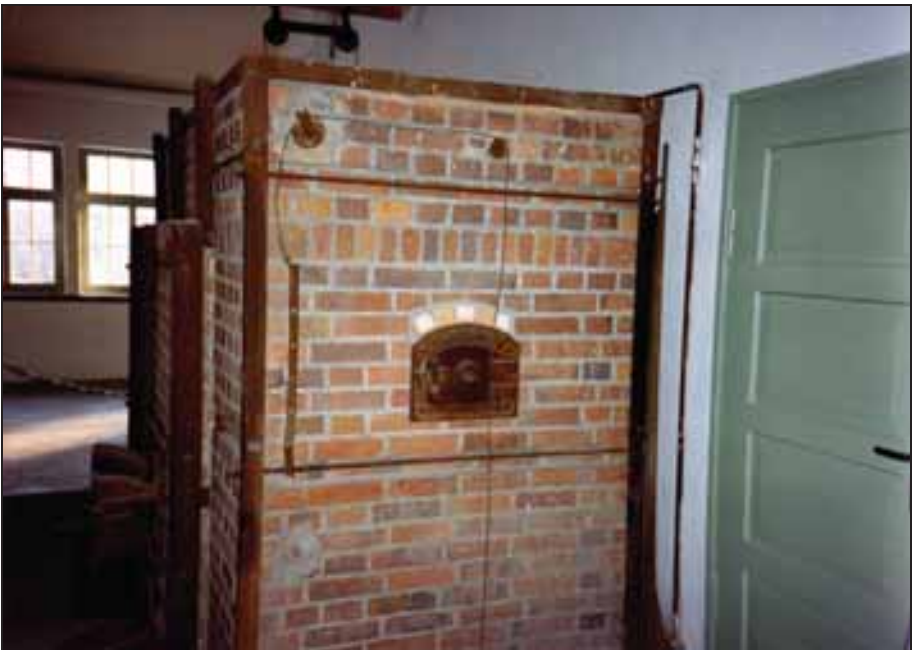
Photograph 259: Rear view of the first furnace; inspection door of the vertical smoke duct. Wire and pulleys for operating the smoke-duct damper, visible in Photo 258 on the floor at the bottom of the furnace.
