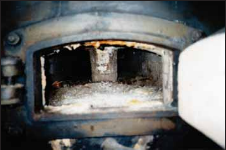
Photograph 354: as above; inside of the post-combustion chamber seen through its rear service door.
