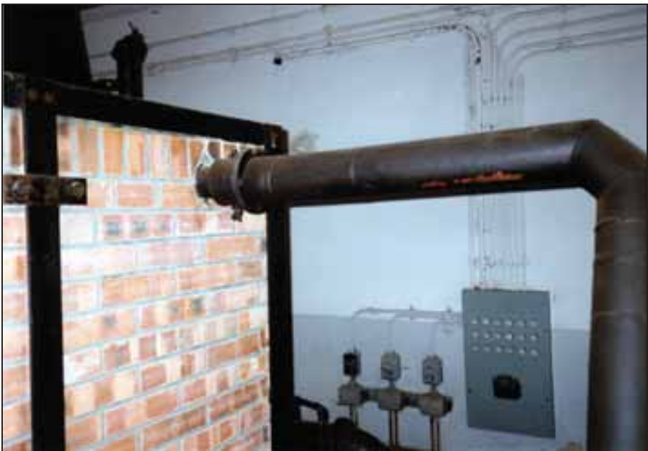
Photograph 192: Blower tube connected to the furnace heated with either naphtha or coke. At the tube's end, close to the furnace's wall, sits a valve for regulating the air flow.
