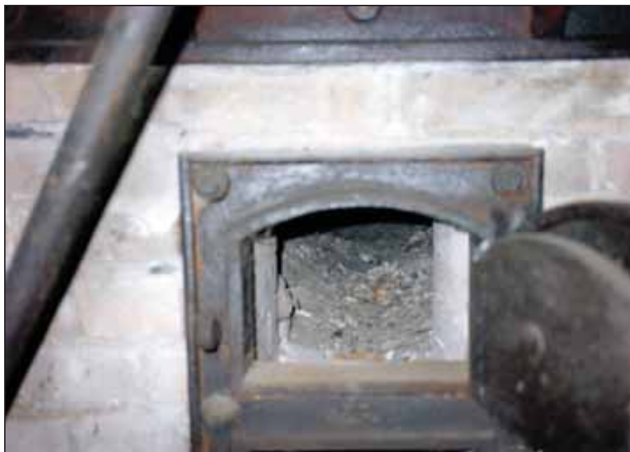
Photograph 303: Access door to the post-combustion area.
