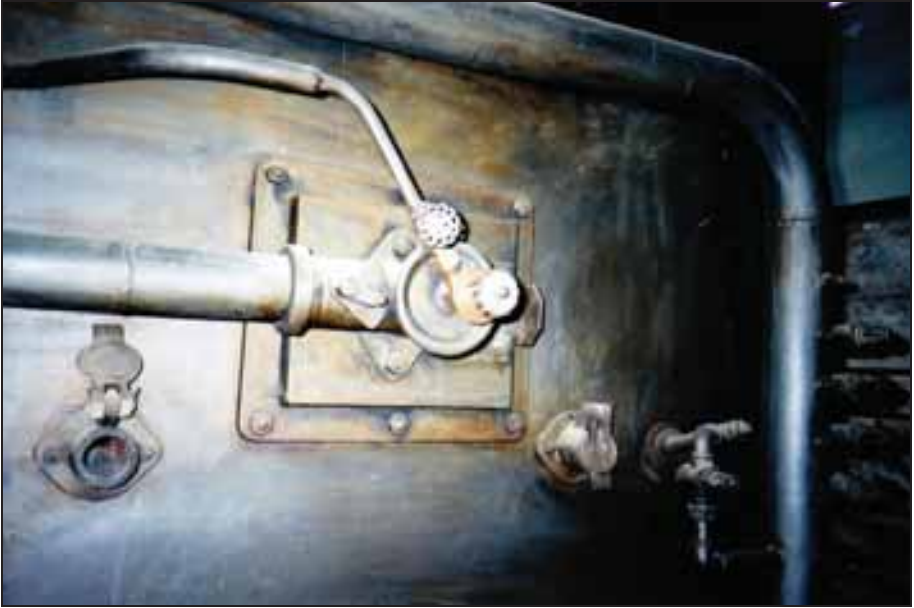
Photograph 350: Right-hand furnace of the front pair, rear view, naphtha burner.
