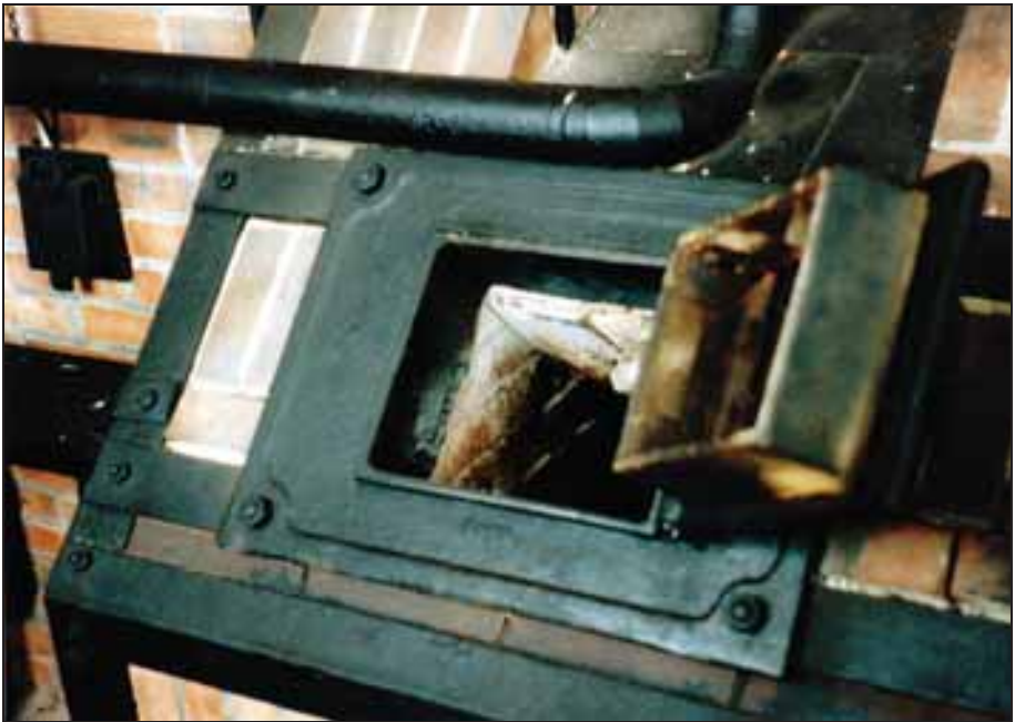
Photograph 162: as above, with opened coke-loading door.
