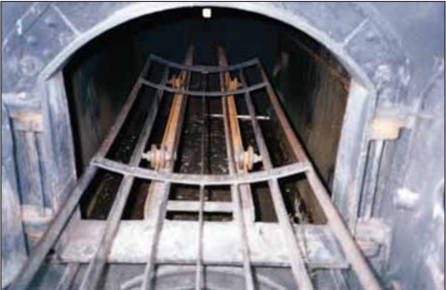
Photograph 334: Interior. The introduction stretcher moved with four metal rollers on two angle irons. The opening in the back wall housed the main burner. The refractory lining has been completely removed.
