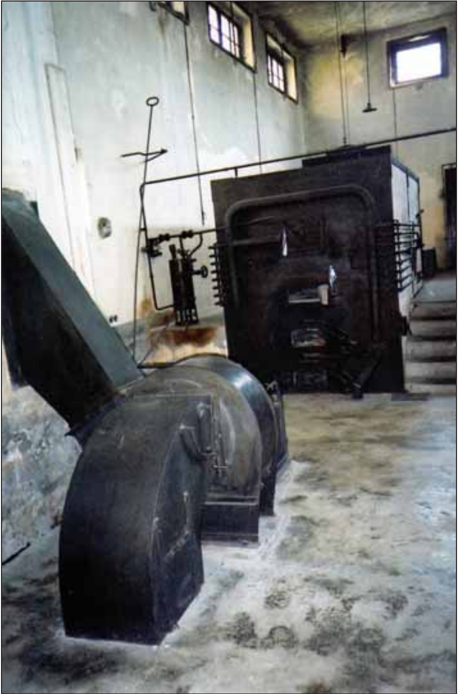
Photograph 357: as above, side view.
