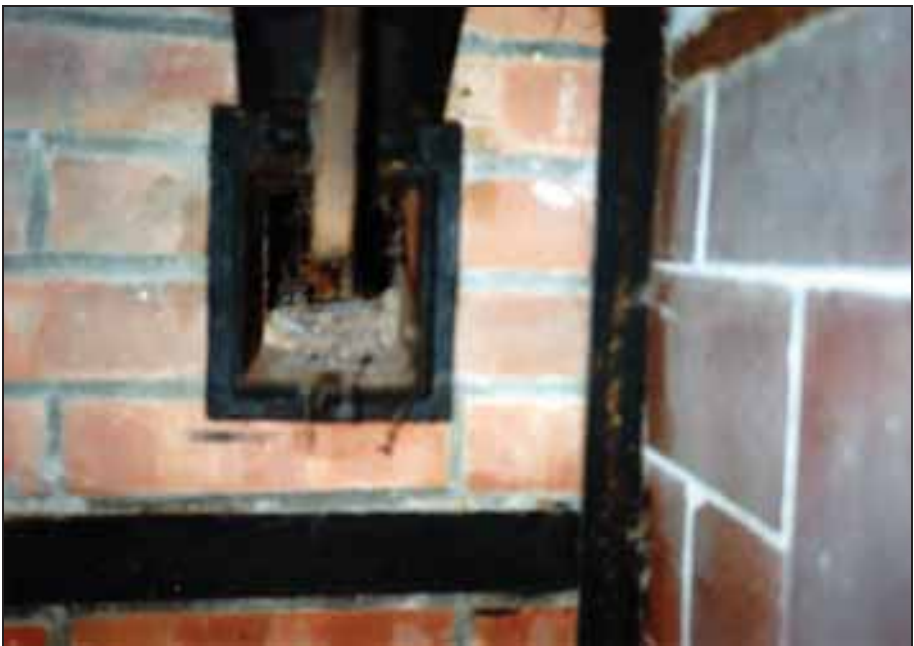
Photograph 166: as above, close-up of the gasifier's combustion-air channel.
