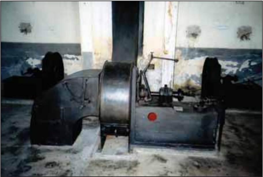
Photograph 356: Forced-draft blower of the front pair of furnaces, with suction duct (left), chimney duct (center) and the motor (right). In the background left and right the two combustion-air blowers.
