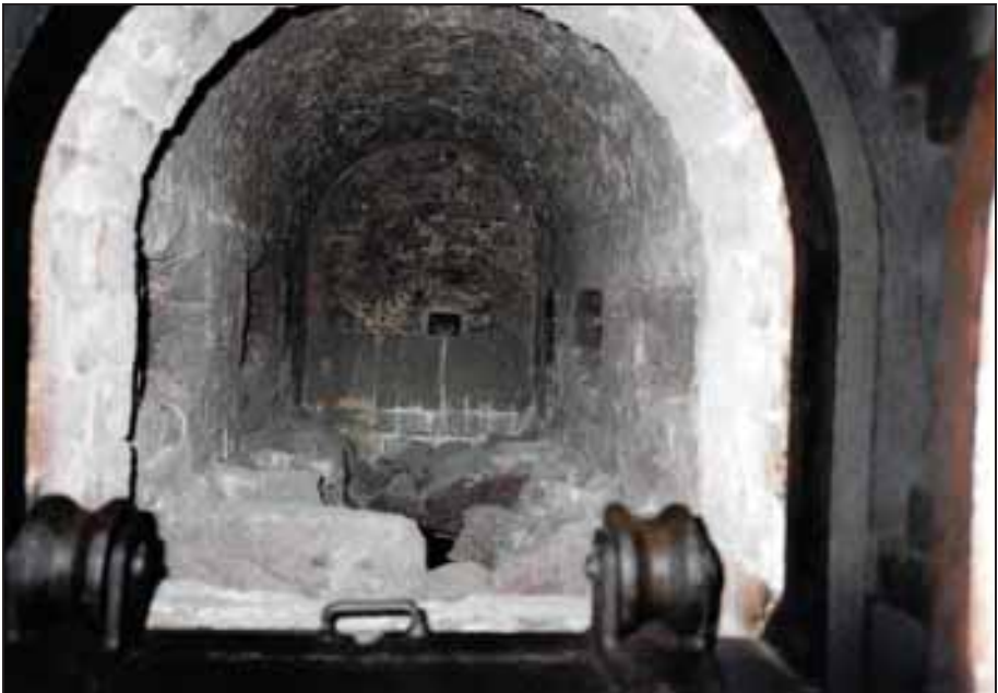
Photograph 180: as above, view into the muffle across the rollers.
