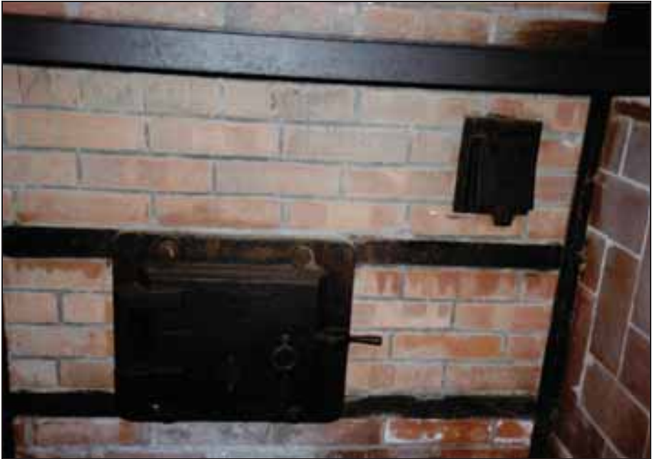
Photograph 165: as above; the gasifier's ash-chamber door (bottom) and the door of the gasifier's combustion-air channel (top right).
