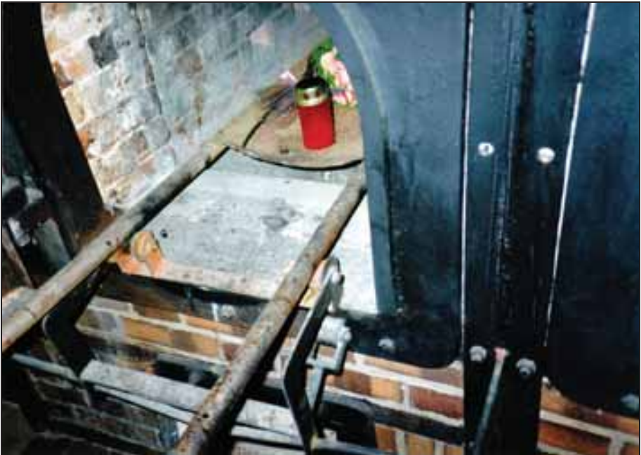
Photograph 85: as above, viewed from top: the movable roller device on which the bars of the corpse stretcher rests.
