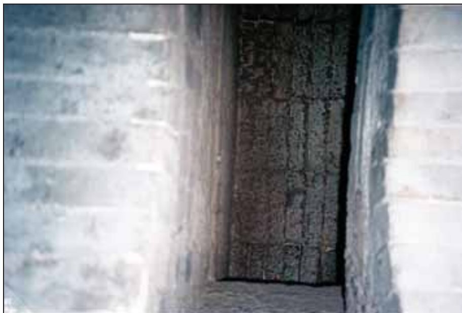
Photograph 302: Vertical duct of the flue-gas outlet.
