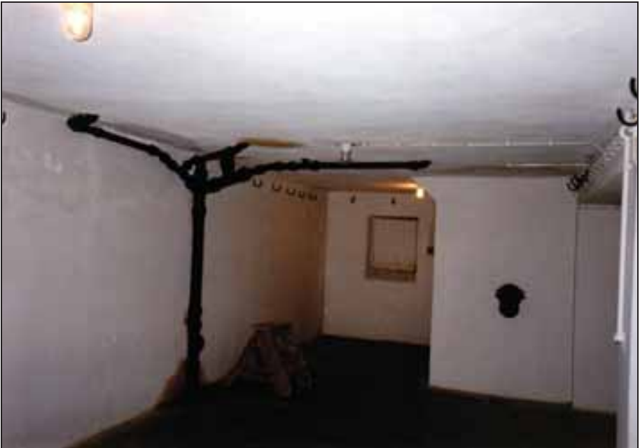
Photograph 211: as above; on the back wall, on the right, the manual controls for operating the freight elevator.
