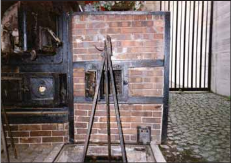
Photograph 8: The furnace's right-hand gasifier with coke-loading door and the gasifier's primary air intake.
