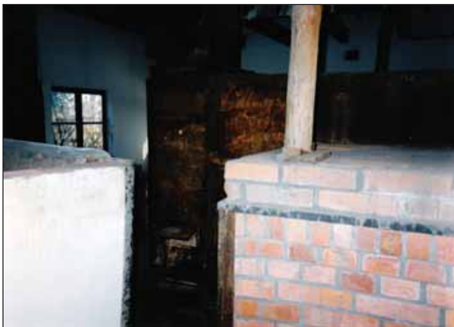
Photograph 50: Left-hand side of the furnace; background: open service door for the pilot flame at the chimney's base.
