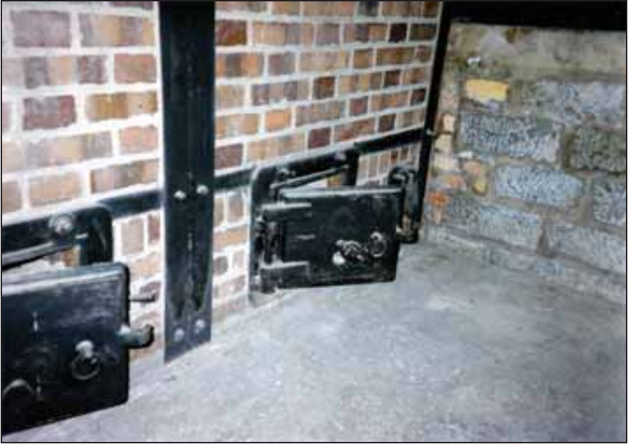
Photograph 80: as above, the gasifiers' ash-chamber doors.
