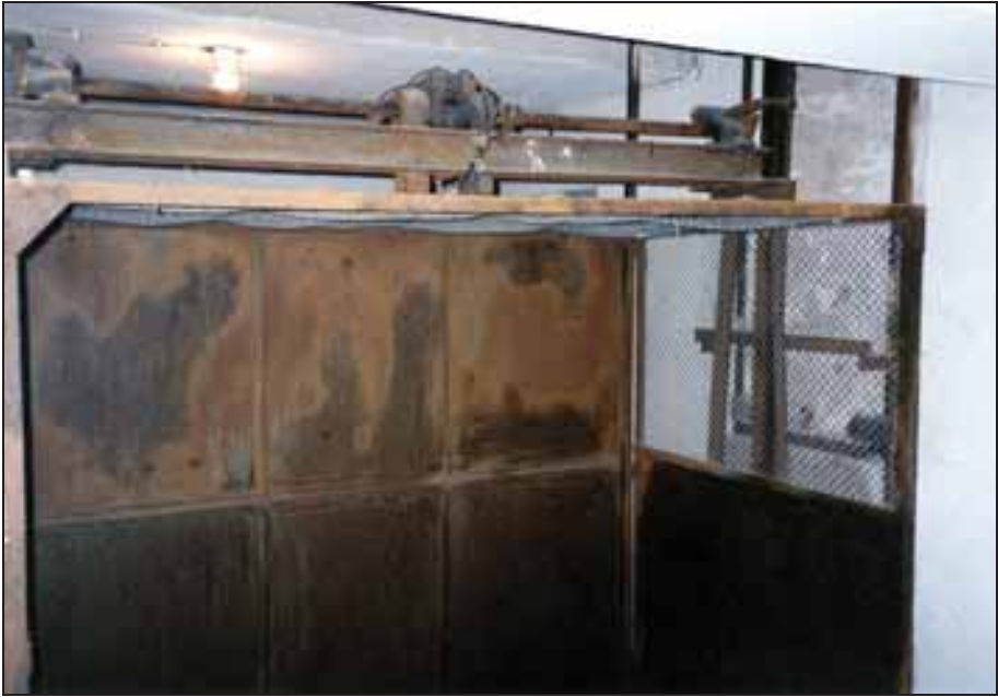
Photograph 212: as above, freight elevator, front.
