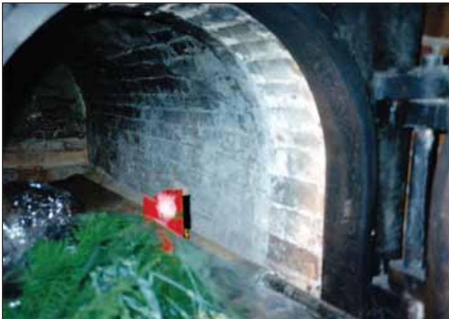
Photograph 55: Right-hand muffle. On the right muffle wall four holes for introducing combustion air can be seen..
