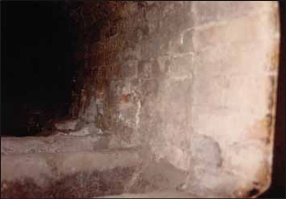
Photograph 147: as above, right-hand square openings of the combustion-air feed. Bottom: muffle grates.
