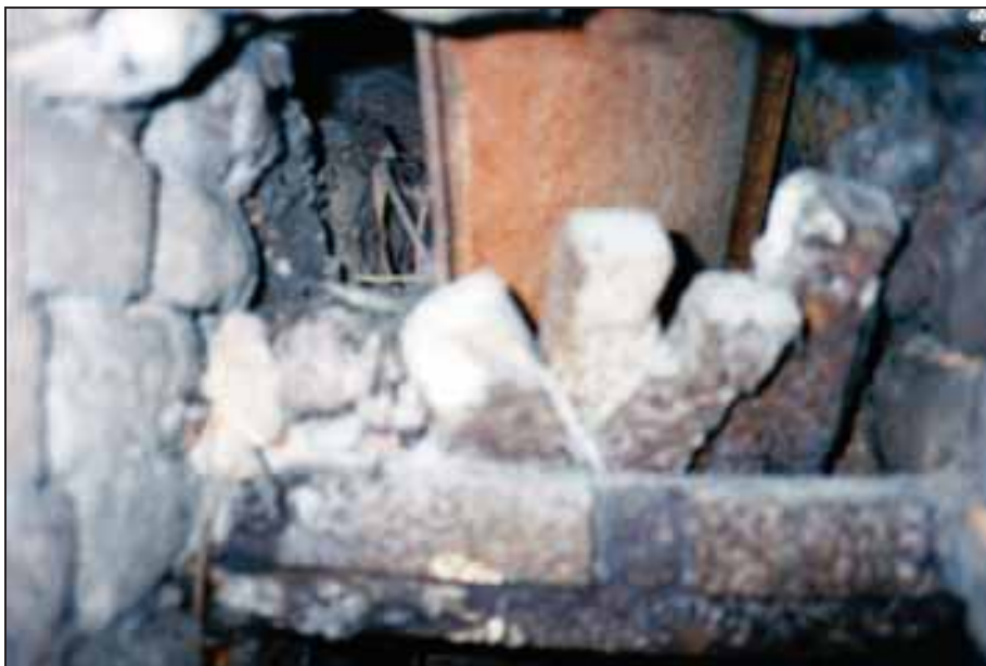
Photograph 277: Inside the right-hand furnace's main gasifier viewed through the ash-chamber door. The hearth's grate has been damaged, with only four remaining bars leaning against the outer support bar.
