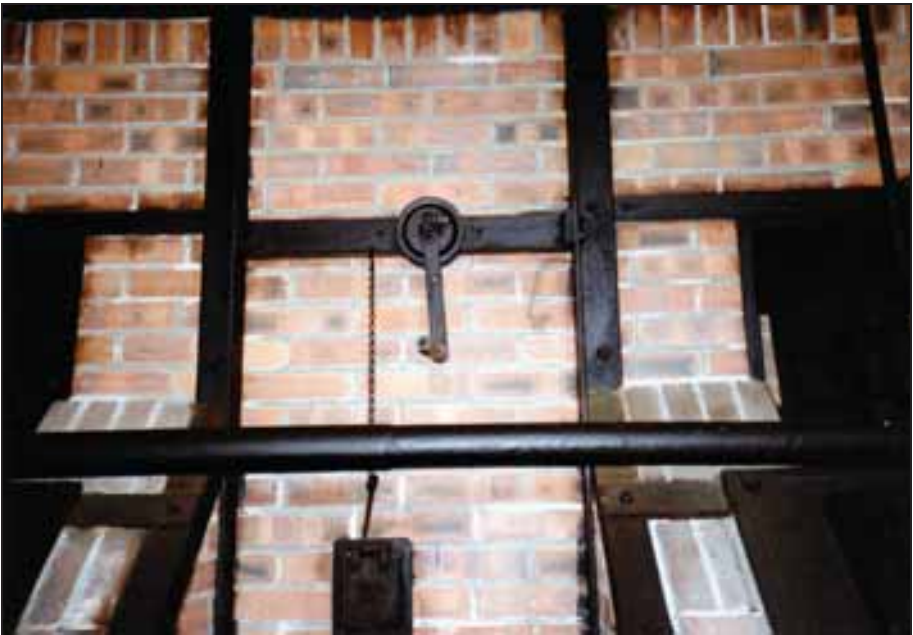
Photograph 168: as above, central muffle. Crank operating the smoke-duct damper (top) and the door to the muffle's rear combustion-air channel.
