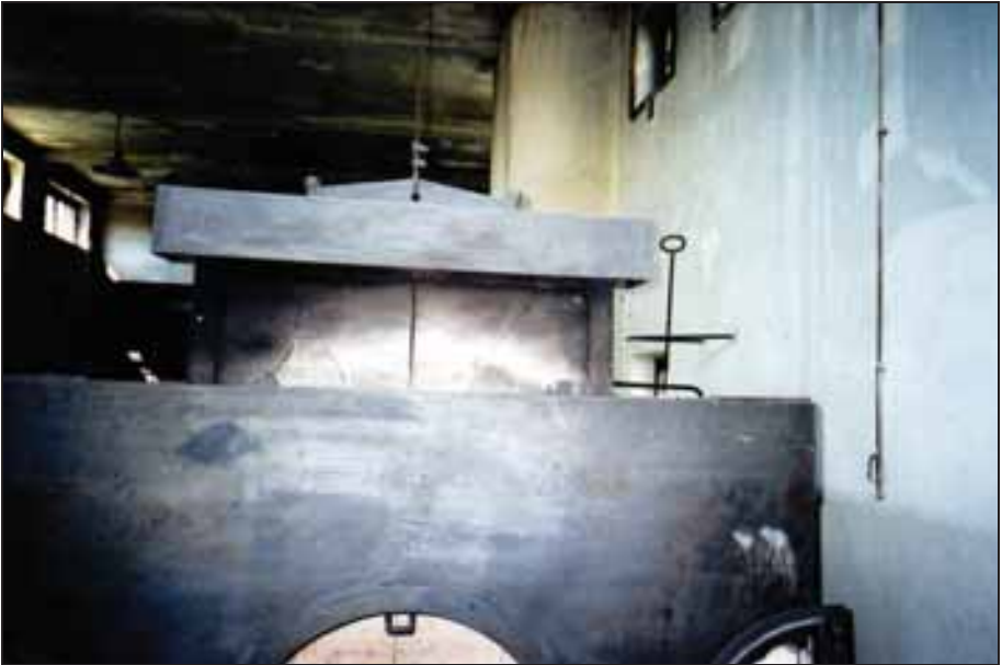
Photograph 359: Closing damper of the right-hand furnace of the rear pair of furnaces.
