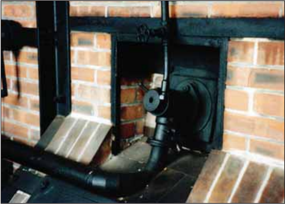
Photograph 204: as above, rear view, naphtha burner of the left-hand muffle; connected to the naphtha burner are from above, the tube feeding oil from the naphtha tank, and from below, the tube from the combustion-air blower.
