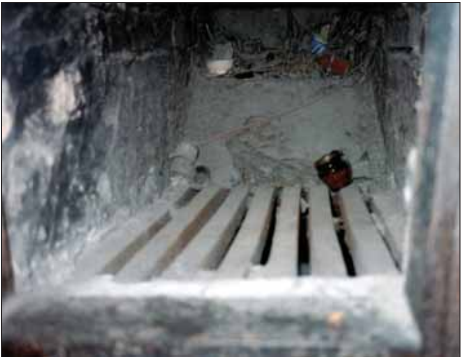
Photograph 99: Furnace 2: original gasifier grate with seven longitudinal bars and two transverse bars.
