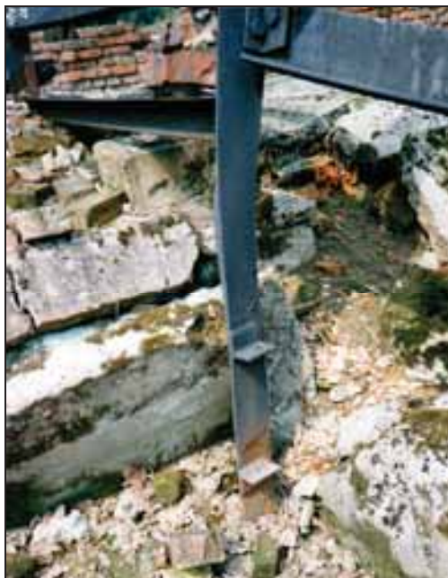
Photograph 231: as above. Detail of the northern gasifier's frame irons (direction south-north). The two brackets visible below were used for mounting the gasifier's hearth door.
