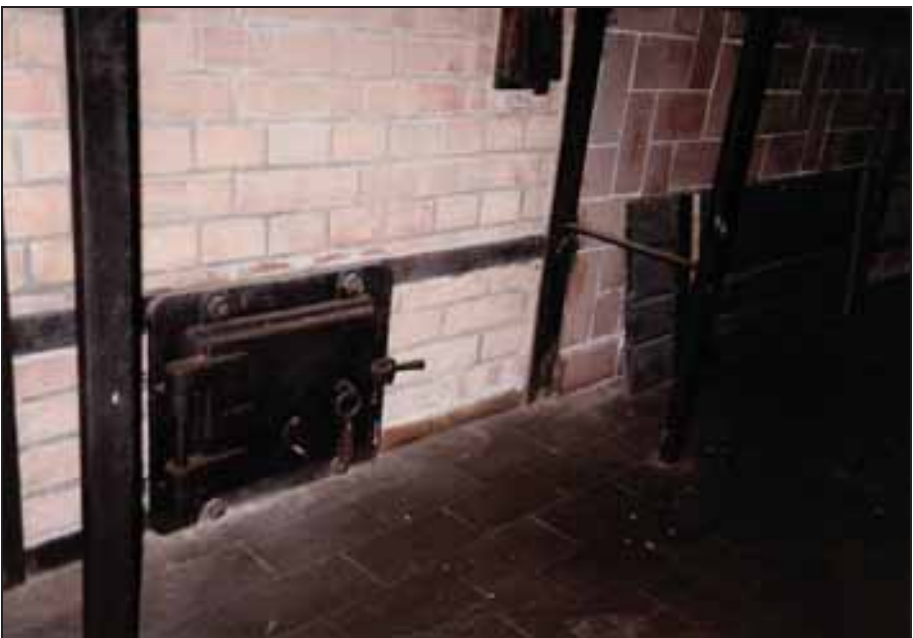
Photograph 176: as above, left-hand muffle: the gasifier's ash-chamber door (bottom) and its combustion-air-channel door (top right).
