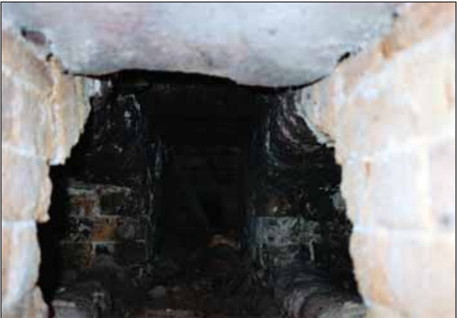
Photograph 156: as above, central muffle's ash chamber with the two lateral openings to the flue duct and a combustion-air-supply hole in the back.
