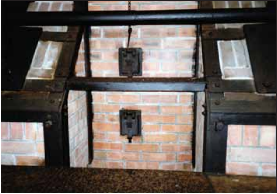
Photograph 169: as above; doors to the muffle's (top) and the ash chamber's combustion-air channel (bottom).
