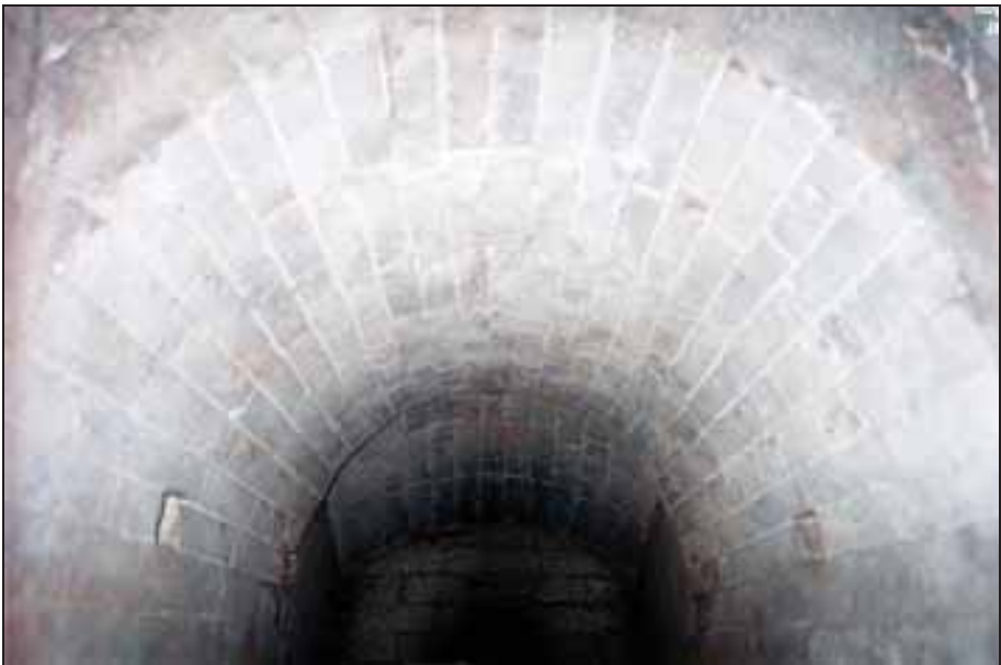
Photograph 297: Vaulted ceiling of the first muffle; in the side walls the openings of the combustion-air-supply channels can be seen.
