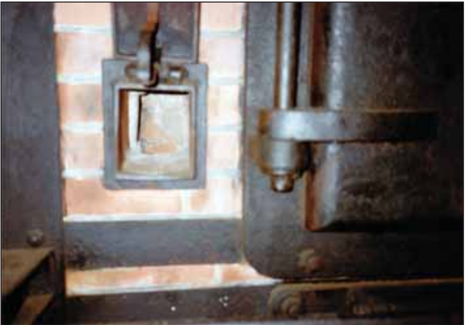
Photograph 152: as above, the ash chamber's combustion-air-supply channel.
