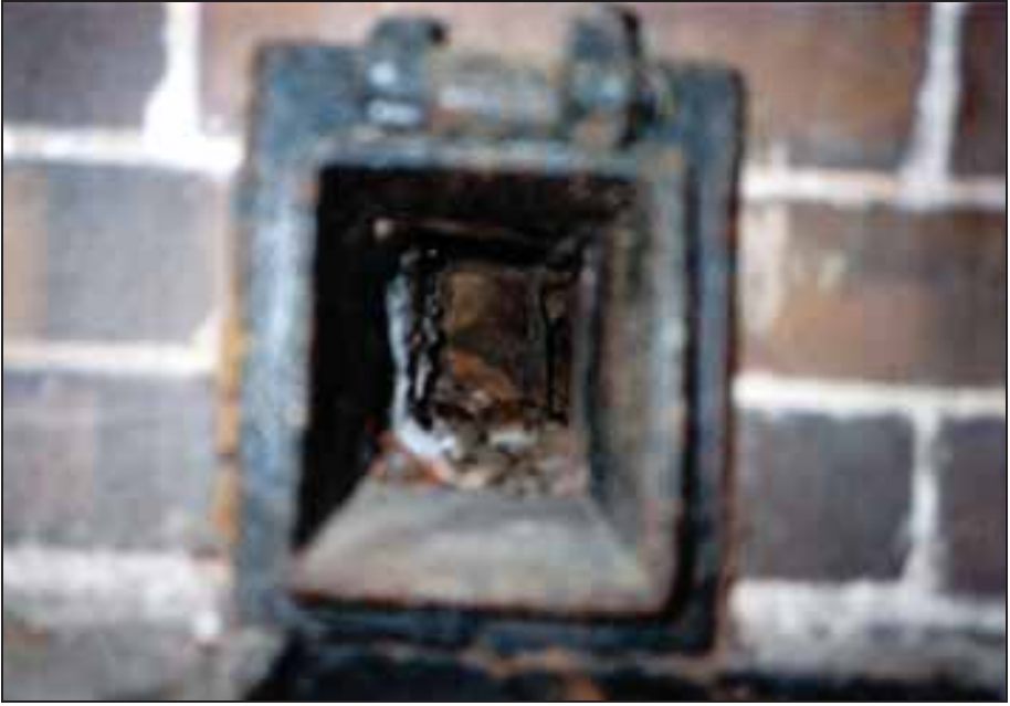
Photograph 6: Left-hand gasifier's primary air intake.
