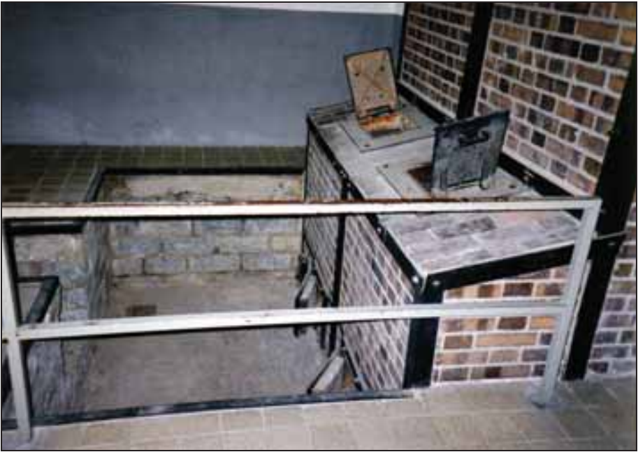
Photograph 77: Rear side of the furnace with the gasifiers and service pit.
