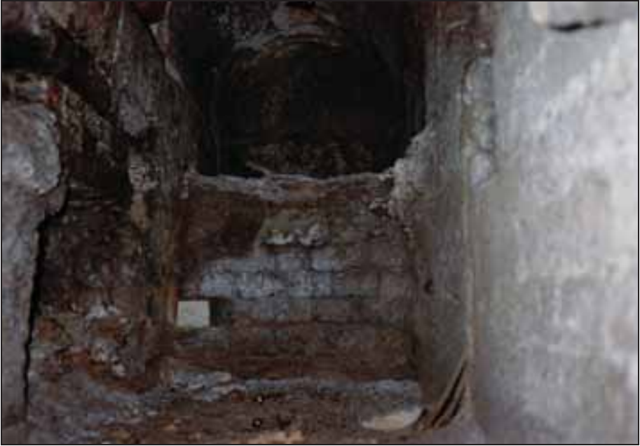
Photograph 18: Left-hand muffle: ash compartment. Visible at the bottom left is the first opening connecting it to the gasifier.
