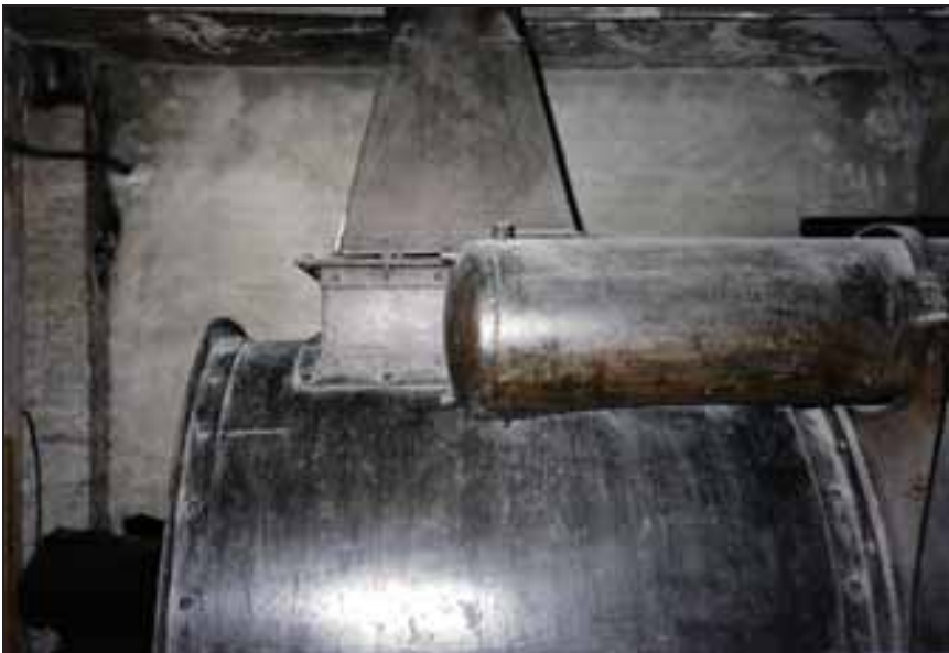
Photograph 331: Right-hand side of the furnace with the naphtha tank in the foreground.
