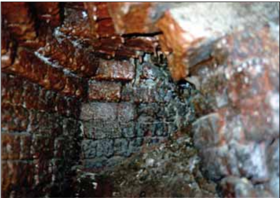
Photograph 5: Left-hand gasifier: Inside view, with the first opening connecting it to the left-hand muffle. The refractory brickwork shows evidence of fusion.
