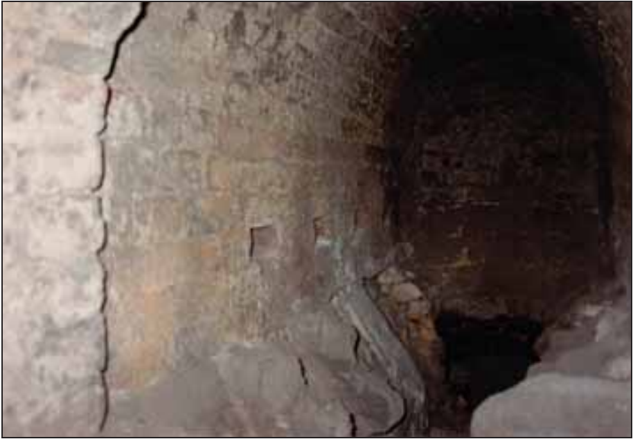
Photograph 141: as above, left-hand muffle wall sloping into the ash chamber with bottom rear opening into the gasifier.
