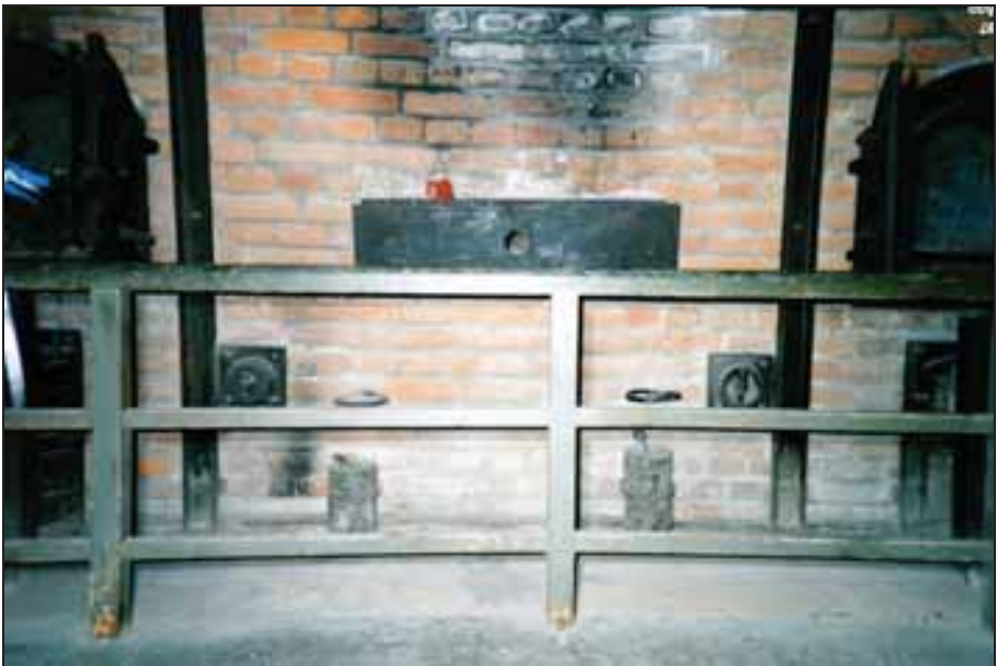
Photograph 289: as above; first recuperator.
