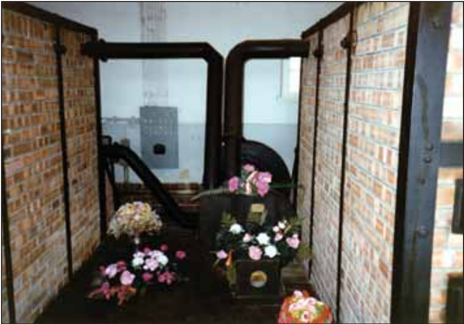
Photograph 188: Blowers located between the two furnaces.
