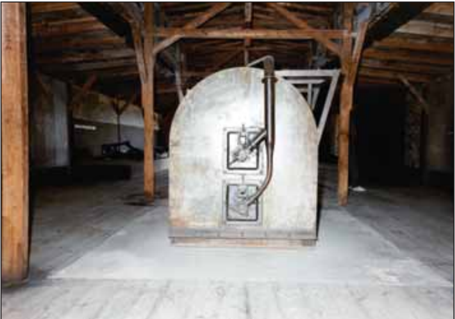
Photograph 327: rear view; combustion-air pipe with main (top) and auxiliary burners (bottom).
