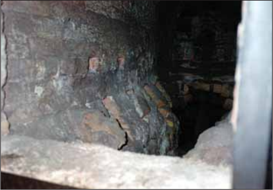
Photograph 131: as above; in the left-hand wall four openings of combustion-air channels are visible; below this the remnants of the muffle-grate bars and the walls slanted toward the ash chamber; in the back at the bottom is the opening to the gasifier.
