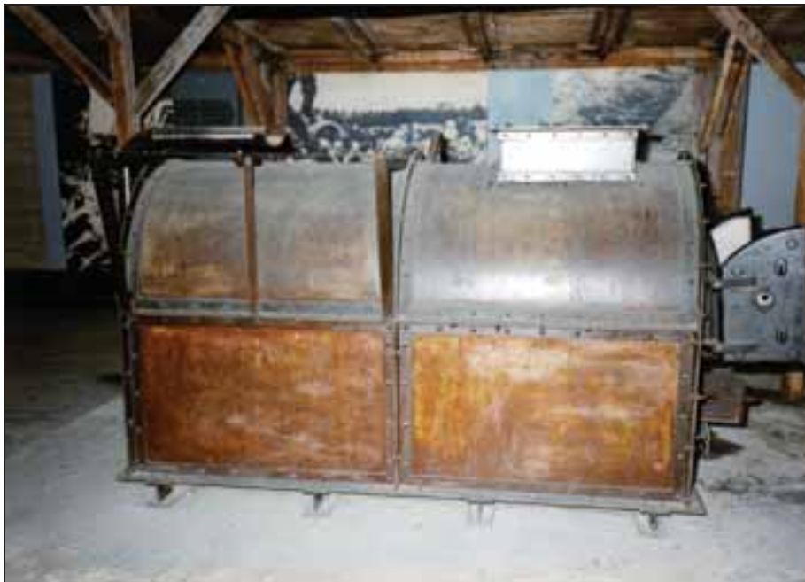
Photograph 325: as above. In the upper part of the furnace can be seen the combustion-air pipe for the burners (left), the support bars for the fan and its motor (center), and the base of the chimney (right).
