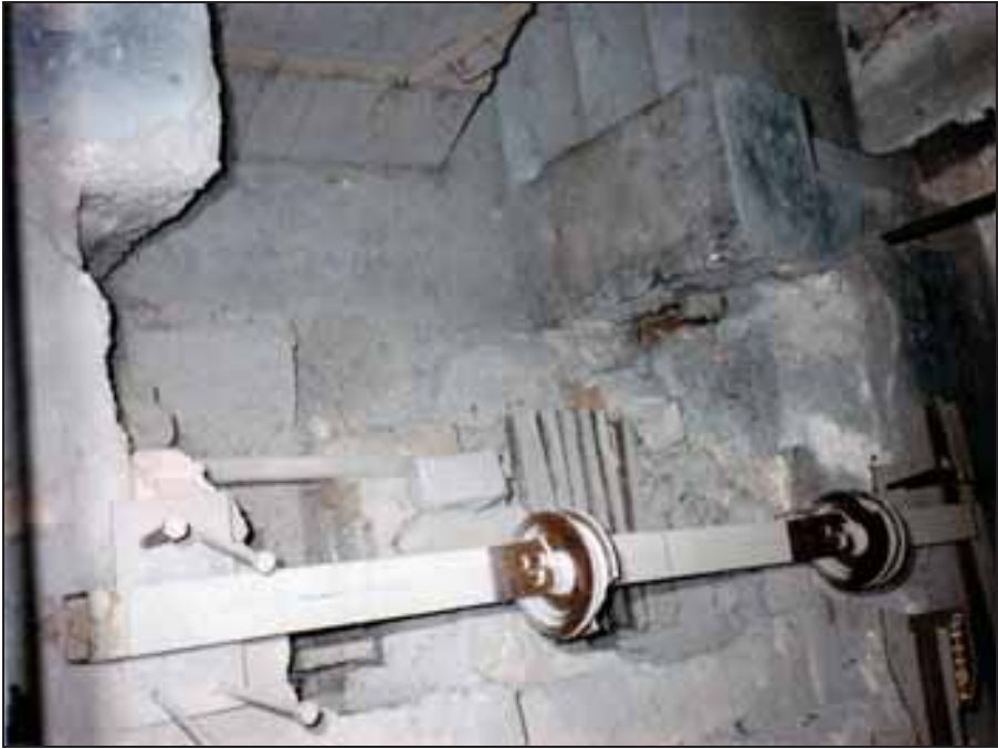
Photograph 100: Ruins of the foundations of Furnace no. 3: service pit and the gasifier hearths seen from the top.
