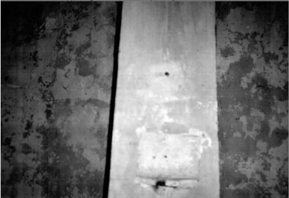
III. 12: Morgue of Crematorium I at Auschwitz. One of the blocks set into the center of the supporting beam of the ceiling. October 1991. © Carlo Mattogno.
