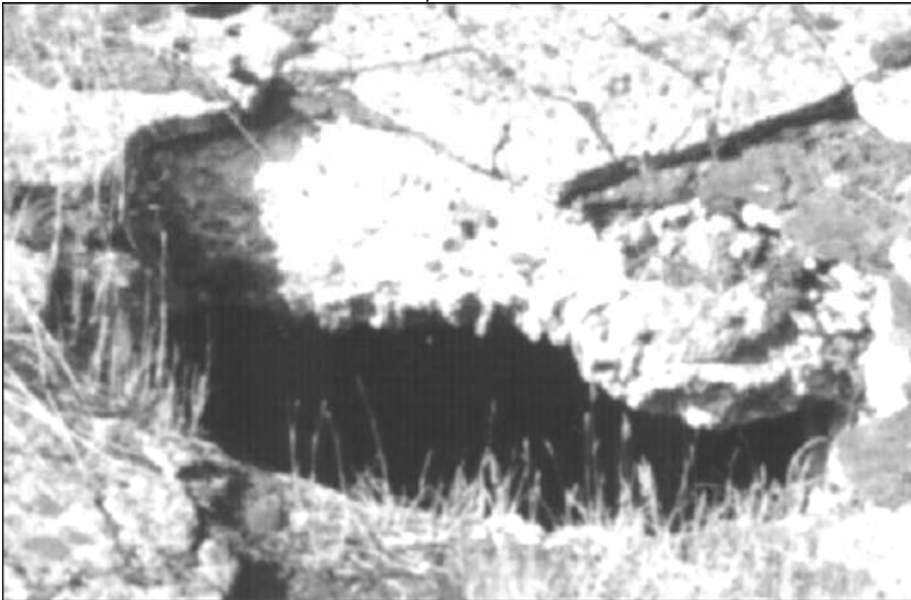
III. 20: Concrete roof of morgue 1 of Crematorium II in Birkenau. Provan's opening 2 in July 1992. © Carlo Mattogno
