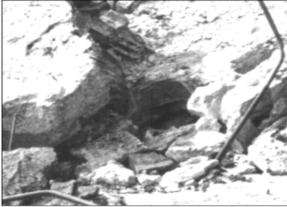
III. 10: Round opening for the pipe of the ventilation through the reinforced concrete roof of morgue 2 of Crematorium II in Birkenau. Section enlargement of III. 9. © Carlo Mattogno
