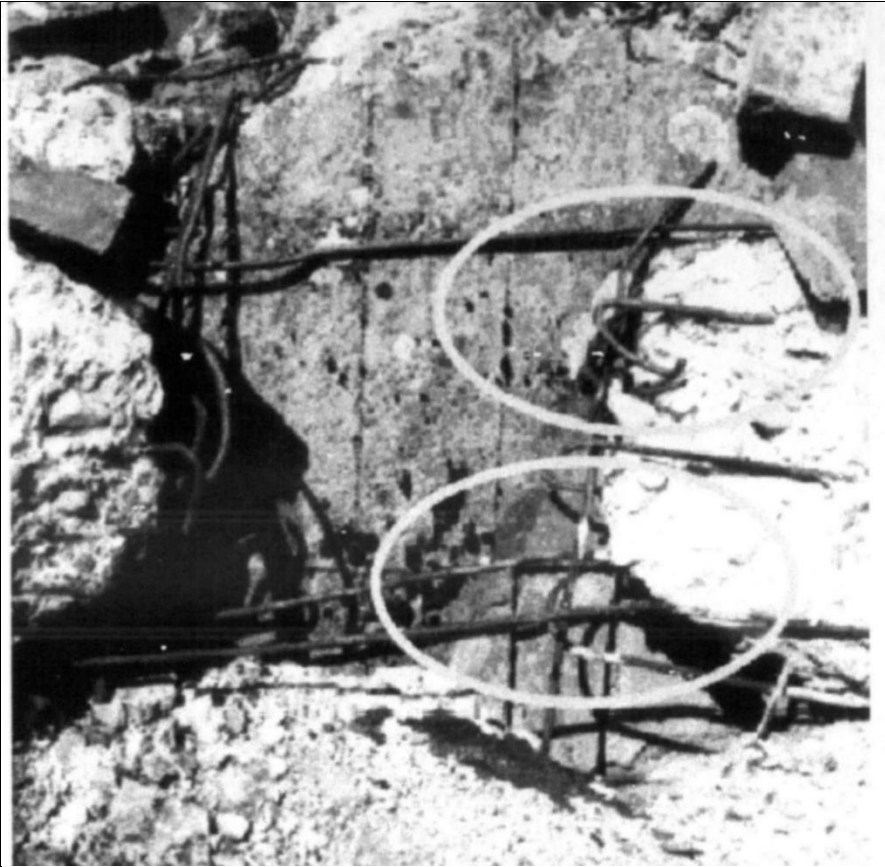
Illustration 22: Collapsed concrete roof of Morgue #1 of Krema II in Birkenau. Keren's opening #4. From Keren et al. (2004: 85)
