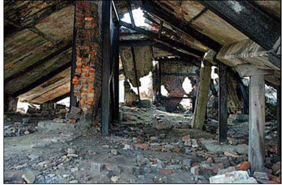
Illustration 14: Under the collapsed roof of the furnace hall of Krema II, Auschwitz-Birkenau.
