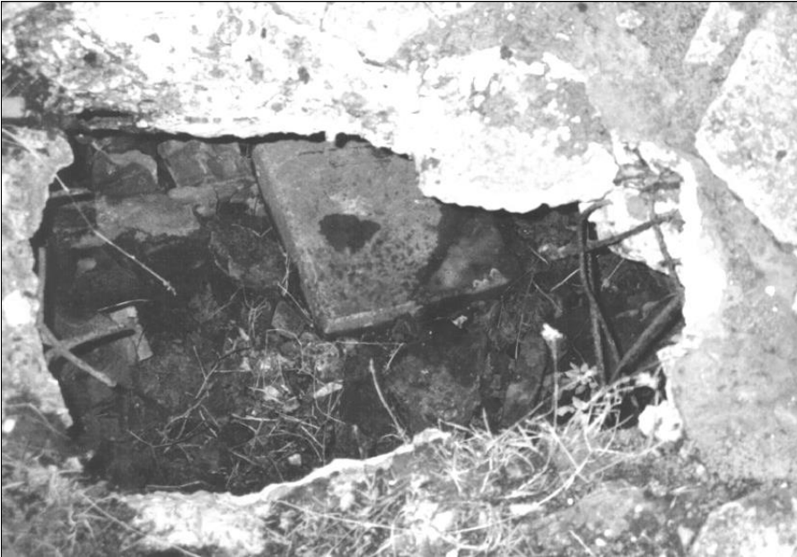
Illustration 19: Collapsed concrete roof of morgue #1 of Krema II in Birkenau. Provan's opening #2 in October 1991. © Carlo Mattogno; from Rudolf/Mattogno (2017: 349)
